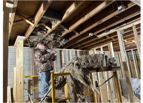
Above: PHS hired Berlin handyman Randy Koscher to stuff insulation and install drywall.
